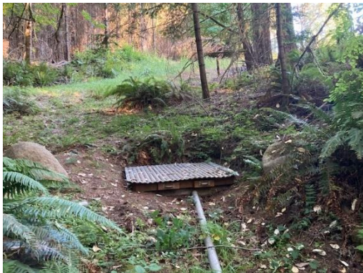
Water source with spring box and overflow pipe; not under direct influence of surface water source.
